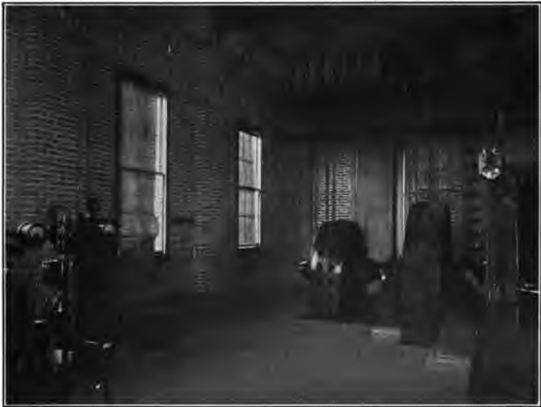
400 H. P. INDUCTION MOTOR DRIVING HOIST AT ATHENS MINE. MOTOR PANEL AND AUXILIARY AIR COMPRESSOR AT THE LEFT AND CONTRACTOR PANELS MOUNTED ABOVE THE HOIST MOTOR.
